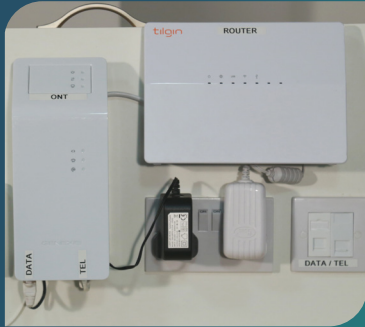
ONT/Genexis, Tilgin router, Power socket.
